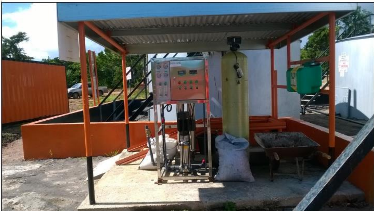
Example water treatment facilities
